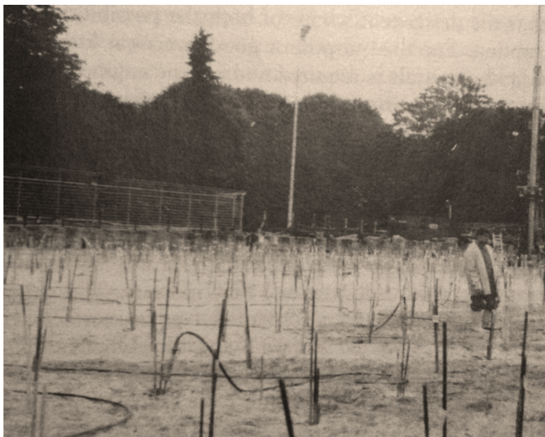
Figure 2.2 Single port grout pipes used in the foundation work for the new Offices of the German President of State (Semprich and Stadler, 2002)
