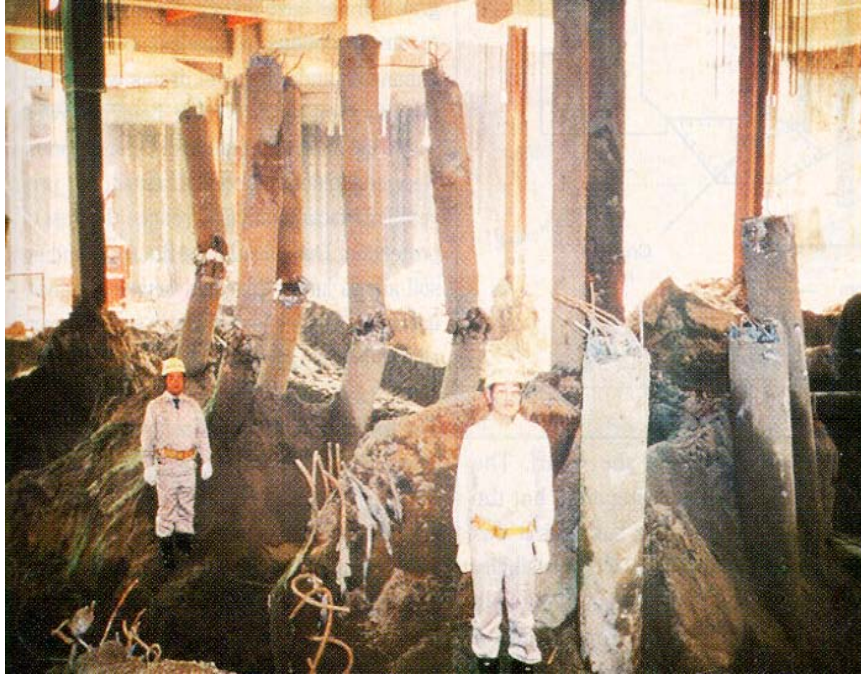
Figure 1.5. Piles supporting the NHK building sheared by lateral spreading during the 1964 Niigata earthquake (Hamada, 1991)
