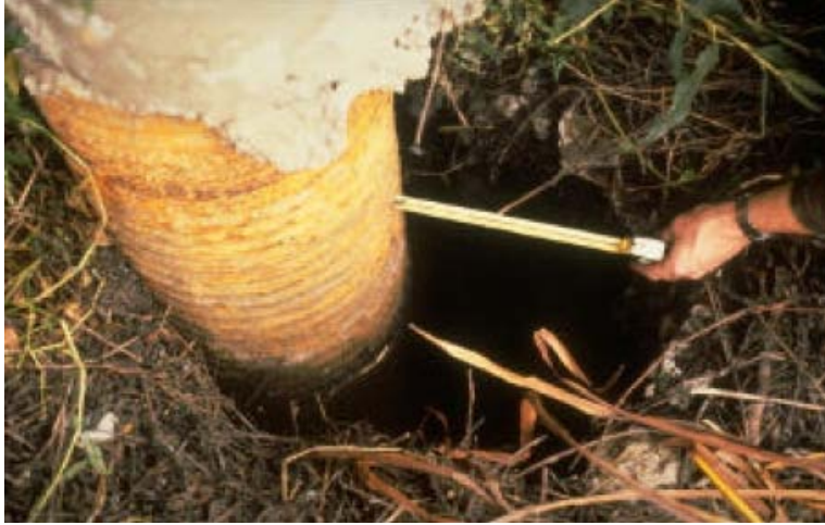
(a) Gap formation adjacent to one of the piles
